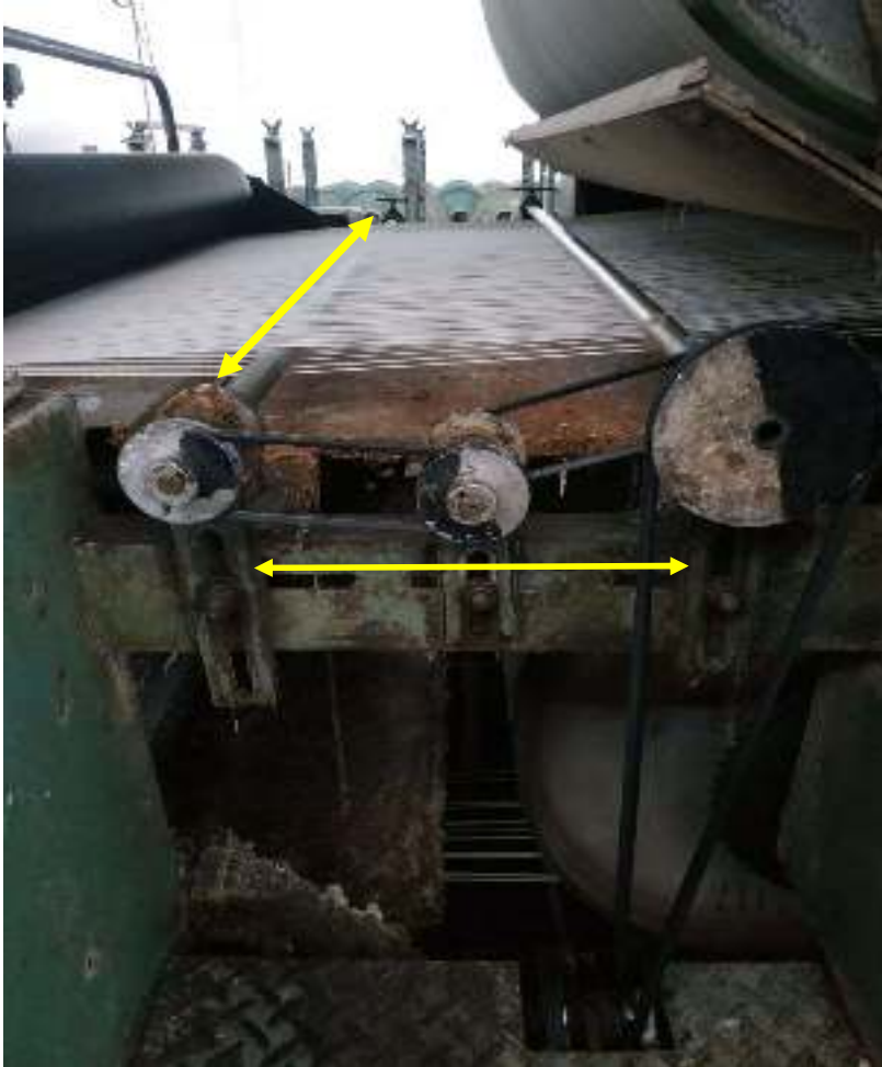
Sumber: unit weaving bagian preparation, 2020
